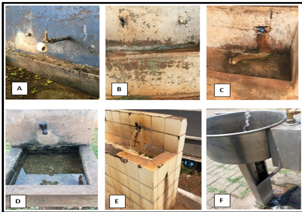
Figure 2. Public drinking fountains with maintenance and physical structure that were considered inadequate: (A) Drinking fountain with the presence of dirt (organic matter); (B) and (C) Drinking fountains with no maintenance and made of brick; (D) Drinking fountain with standing water; (E) Drinking fountain damaged with lateral water leakage and (F) Drinking fountain damaged.
